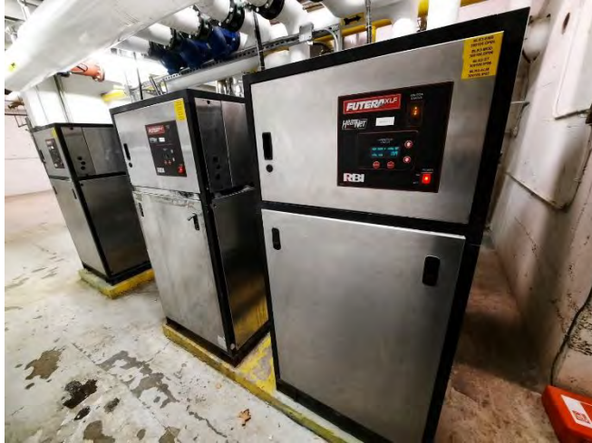
Photo 9: View of the natural gas-fired hot water heating boilers, located in the boiler room of the Subject Building.
