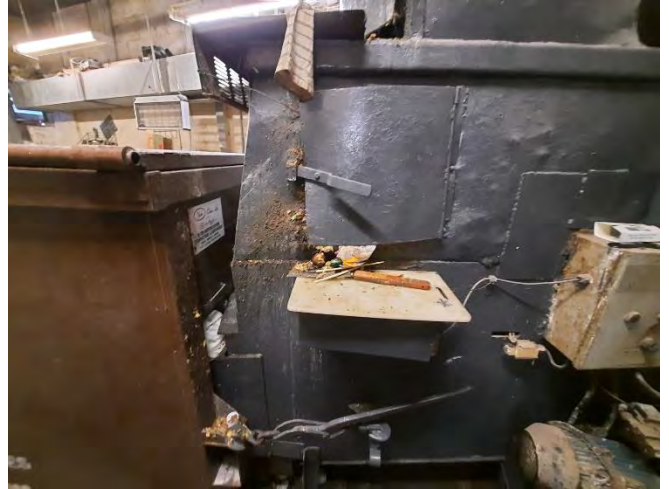
Photo 10: View of a portion of the garage compactor in the garbage room of the Subject Building.
